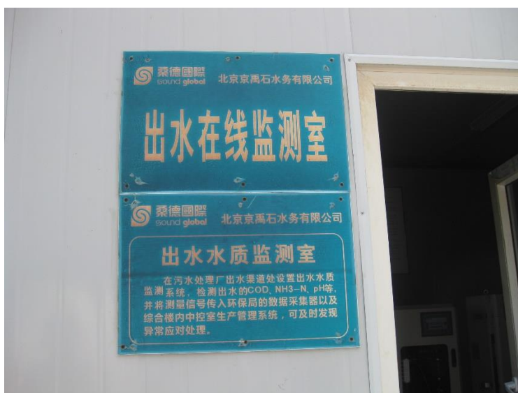
Figure 5: 五里坨污水处理厂在线监测室和设备
